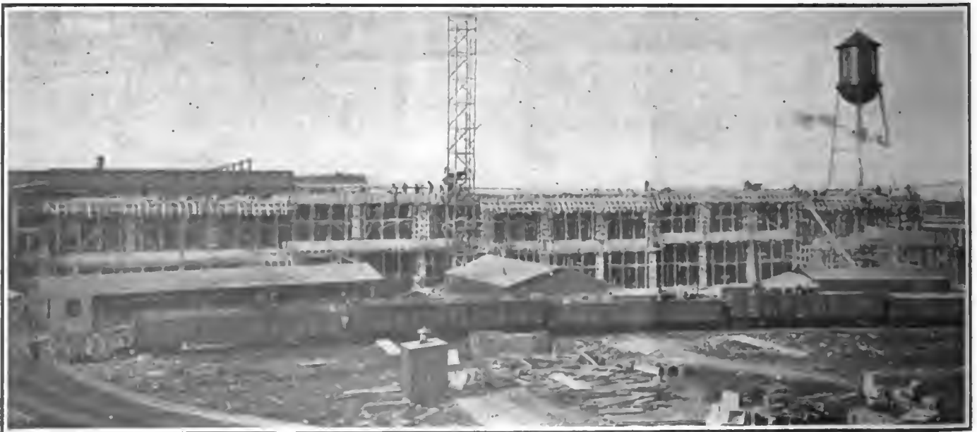
Giving an idea of the size of the new storehouse and assembly building. To carry materials used in the new buildings it was necessary to run two lines of railroad track into the Pierce-Arrow yards. One, with a line of cars on it is shown, the other being in the extreme rear of the site or foreground of the photograph.
